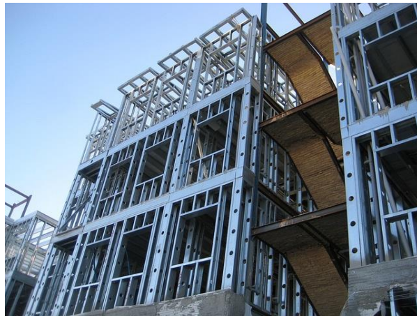
Figure 2.2: Two story residential building entirely built in cold formed members ( https://framecad.com/blog/accelerate-the-construction-of-mid-rise-buildings-with-cold-formed-steel-and-framecad [accessed on November 2024]).
