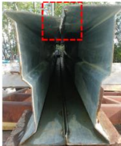
Figure 3.13: Distortional buckling failure in face-to-face sigma section adopted by [77].
