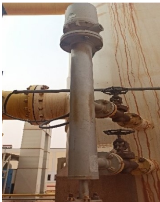
Level Switch High/High sensor
