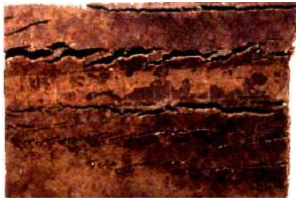
Figure I.12: Fissures de CSC [54].
