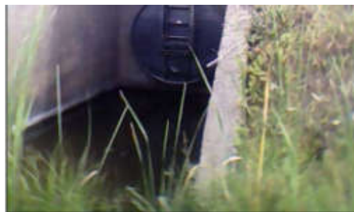
Photo 1. Downstream rejection structure of the canal towards wadi El Kebir (phot. F. Sennaoui)
