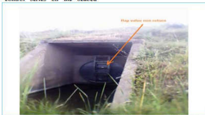
Figure 10. Discharge work under dike leads into El Kebir river canal D03 (photo Sennaoui . F 2016
